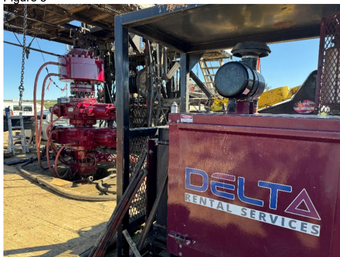
Figure 3 - Surface pressure control equipment (hydraulic accumulator foreground and blowout preventor in the background)
